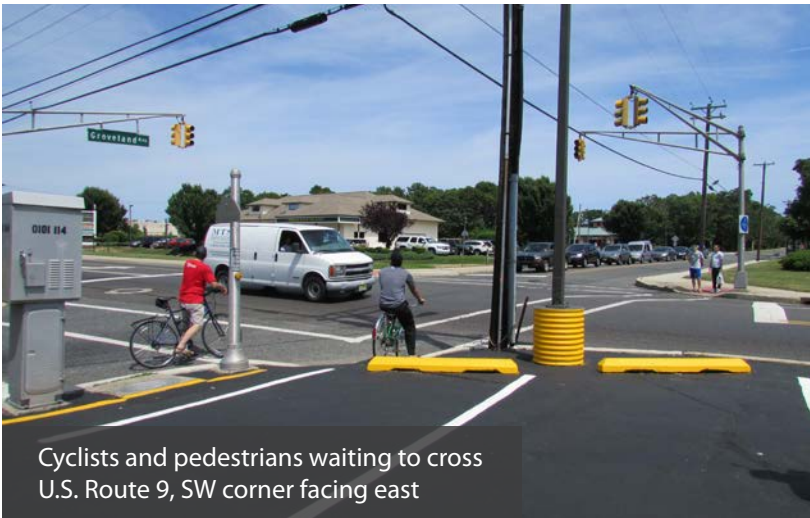
Deficient curb ramp, NW corner
