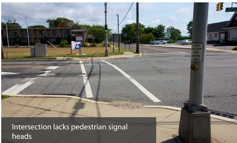
Curb ramp without detectable warning surface, SE corner
